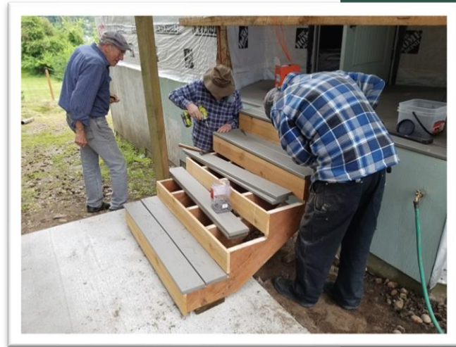
Volunteers Ken Wassum, Paul Michaels and Rick Thompson complete the side stairs
