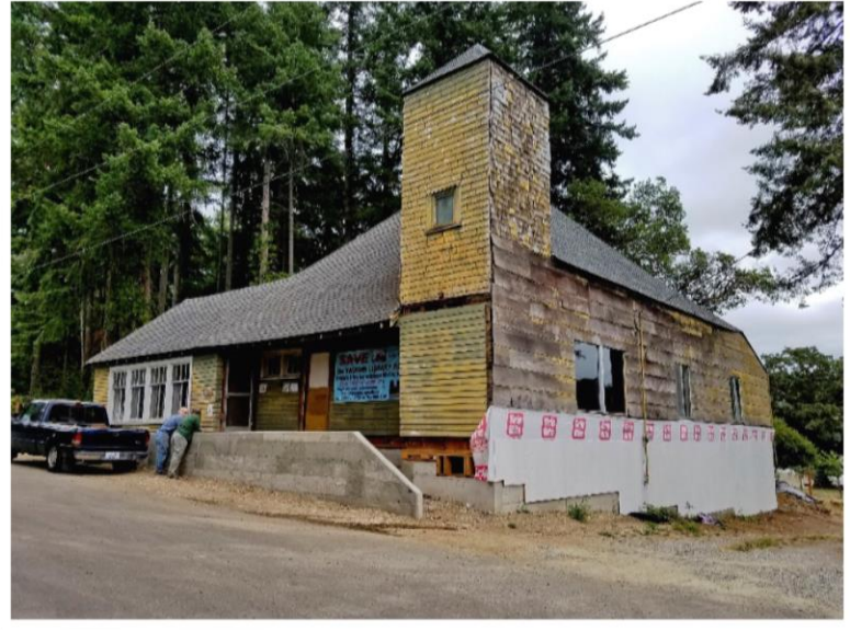
Paul Michaels and Diane Jackman admire the new foundation and plywood sheathing.
